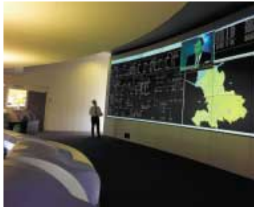
Nuon, Netherlands: Energy Transportation and Distribution Network Center. Barco's solution provides Nuon's operators with all critical information at a glance, reducing the reaction time per event. (Picture courtesy of Nuon, Netherlands)
