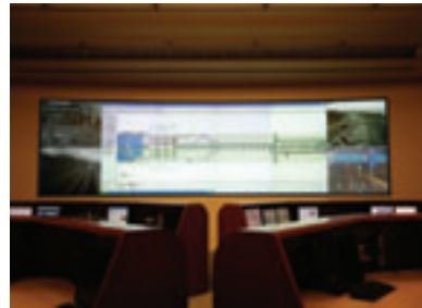
The Utilities Management center
