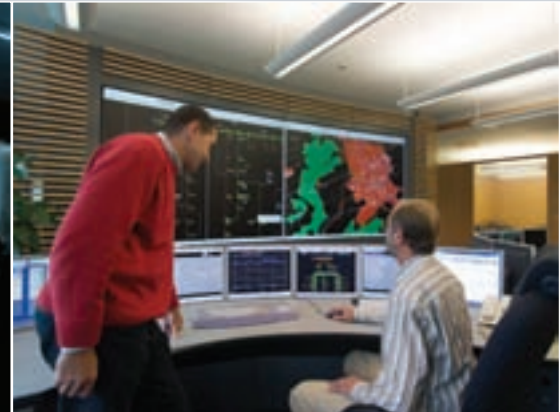
EnBW ZNL Esslingen, Utilities & Process control
